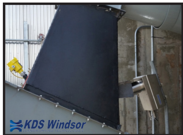
Typical Installation of Green Sawdust Burner System
