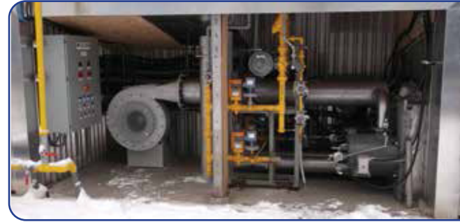
A self contained natural gas heating system that directly drives the steam generator.
